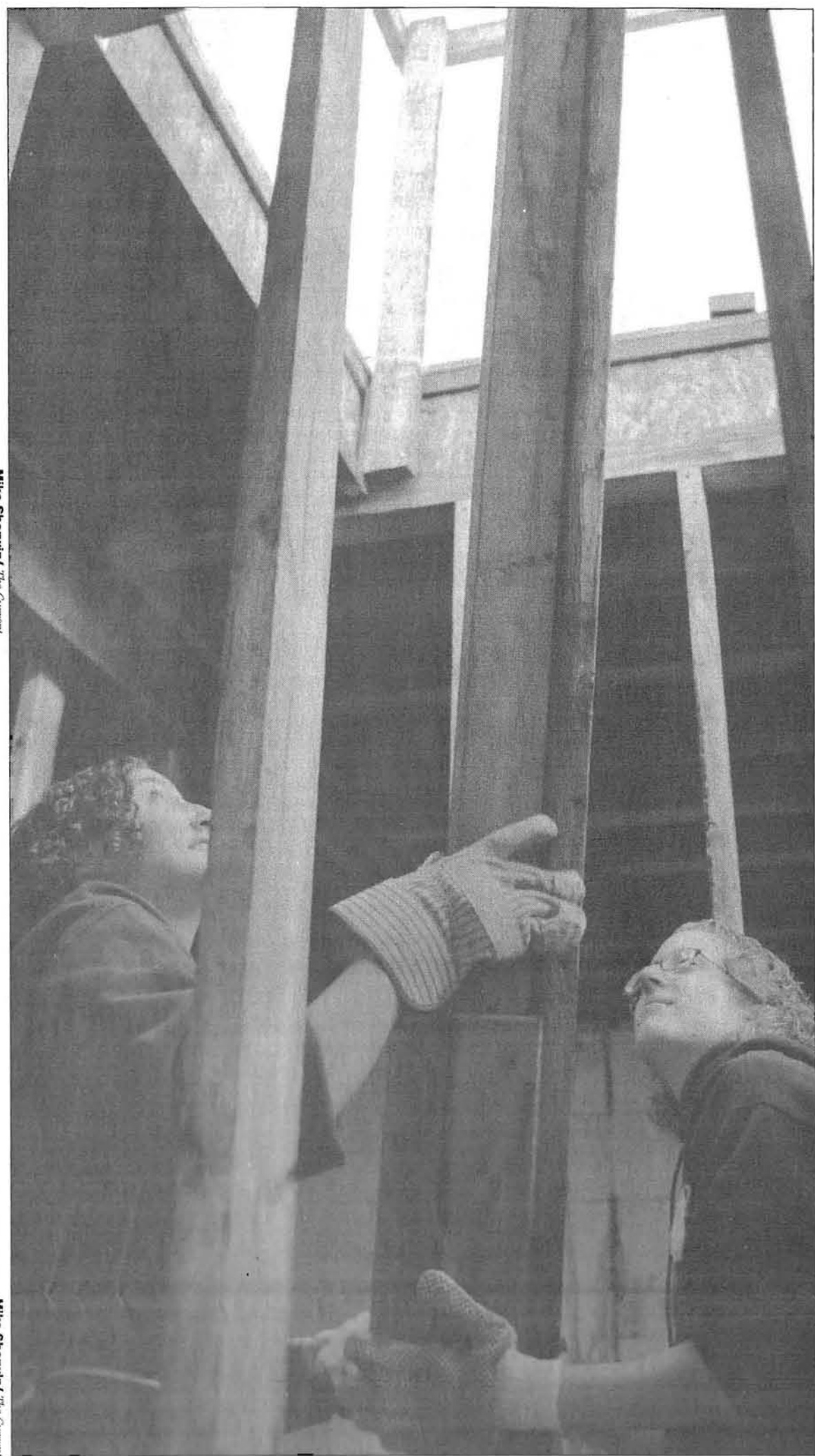
Ashley Mensinger, freshman, graphic design, and Laura Steigerwald, freshman, undeclared, lift a 2x4 to helpers on the roof last Saturday at a Habitat for Humanity site in Wellston.
